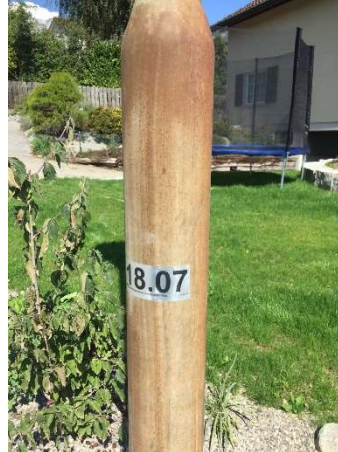
starker Rost am Mast
